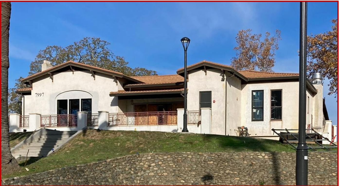
This is what the Community Clubhouse, currently being remodeled, looked like in December, 2024, nearing an early 2025 completion.
